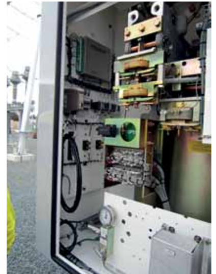
Mitsubishi 120 sfmt 145 KV
